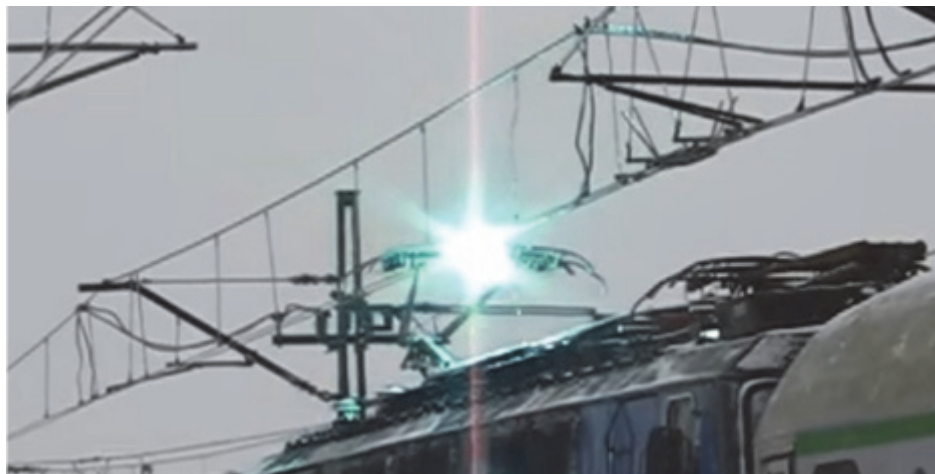
Fig. 2. Electric arc resulted from a ride with a frosted catenary (Kocłęga 9)
